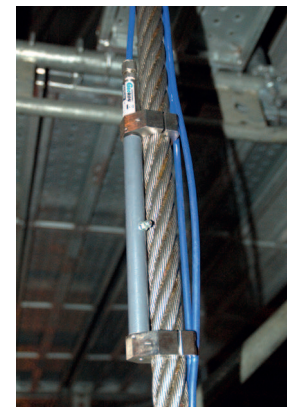
Figure 3: Vibrating wire strand-meter on sling wire.
