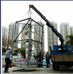
▲ At the Lynwood Sitting-Out Area in Tin Shui Wai, the engineering team used the lifting truck to help installing "Contact"
