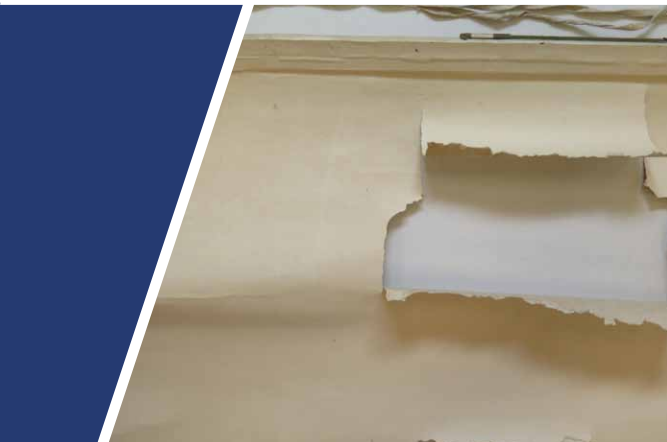
▲ The paper borders showed serious damages and there were cracks near the upper rod
