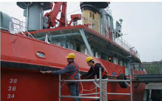
▲ Contractors scraping off corrosion and the deteriorated coating from the fireboat “Alexander Grantham”
