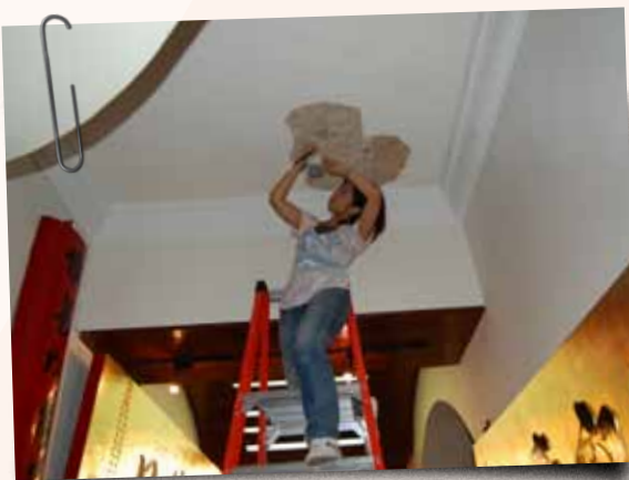
▲ Preserving a century-old newspaper embedded in the ceiling of the Tung Wah Museum
